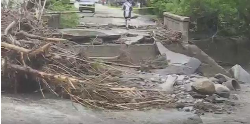
Figure 59. Clip from You Tube video showing damage to Bridge 21 from flooding on May 27, 2011 (You Tube May 2011).
