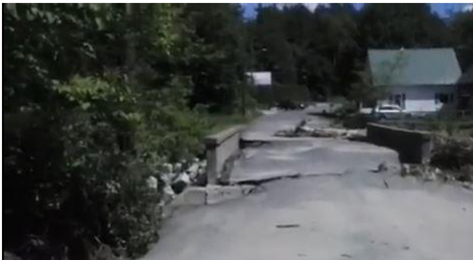
Figure 61. Clip from You Tube video showing damage to Bridge 21 from flooding on July 19, 2015 (You Tube July 2015).
