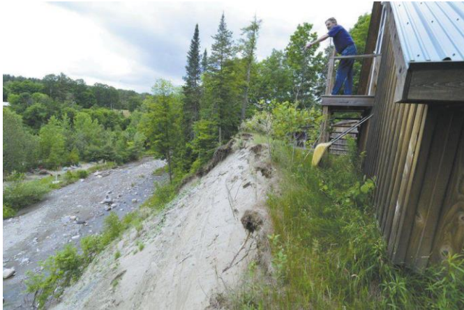
280 Cameron Road was at high risk due to fluvial erosion from the Great Brook. The town received a grant through the Community Development Block Grant in 2017 to conduct a buyout of the property. This included removal of the house, garage, outbuildings, and fuel storage tank on the property.
